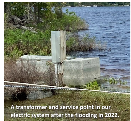
A transformer and service point in our electric system during the flooding in 2022.
