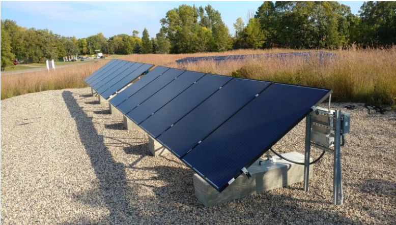
Lake Region Electric Cooperative's 6 kW GoWest Demonstration Solar Pelican Rapids, MN
