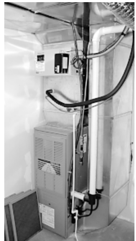
One of the more popular heating systems today is a fully automated, forced air dual fuel system with an electric plenum heater and propane backup.
